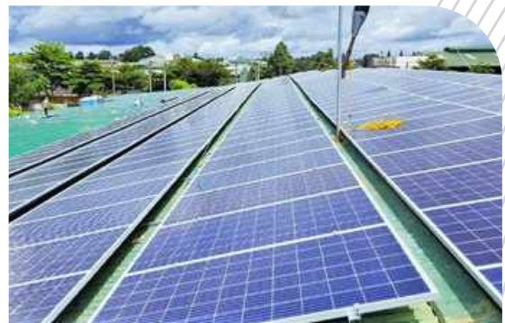
Rooftop solar power project at Phuong Dong company - 560 kWp Location: Dak Lak
