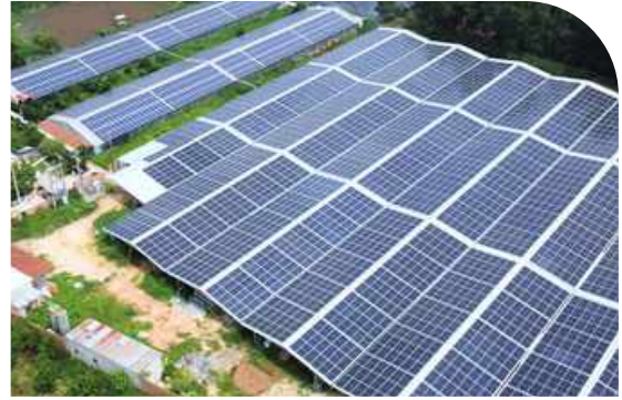
Rooftop solar power project in Dong Nai - 1617 kWp Location: Dong Nai
