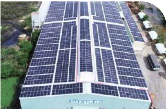
Rooftop solar power project at Muoi Thu packaging factory - 704.94 kWp Location: Binh Dinh
